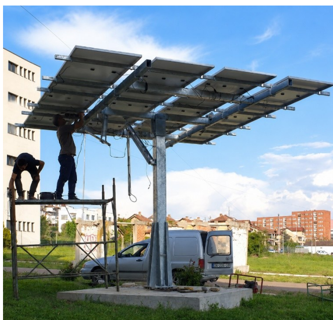
Fig. 17 Final dual-axis solar tracking system
